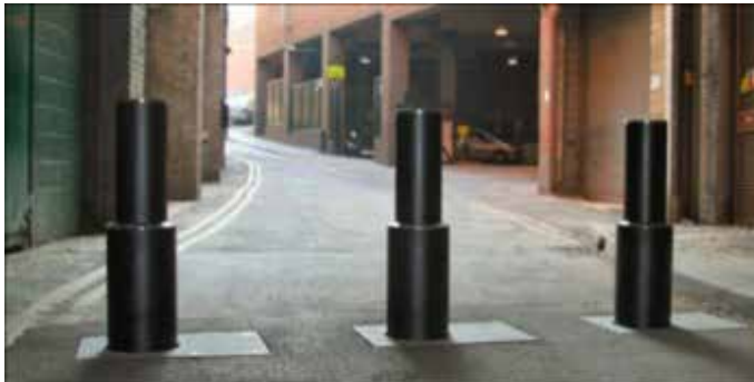
Image 7. Shallow-mounted automatic bollards.
